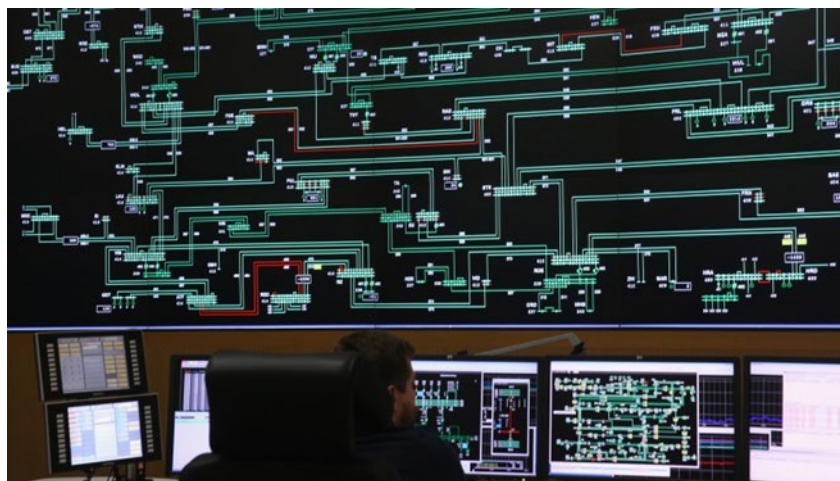
FIG. 2 Incident on the European electricity transmission grid – January 8, 2021 (source: https://www.digi24.ro/stiri/economie/energie/transelectrica )
